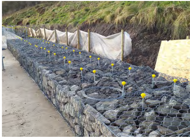
Gabion baskets being built and filled along the side of the promenade
